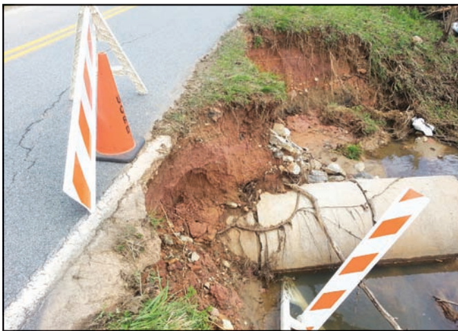
Heavy Rains damaged roads, driveways and culverts in Union County on Wednesday. The county received almost 8 inches of rain.
